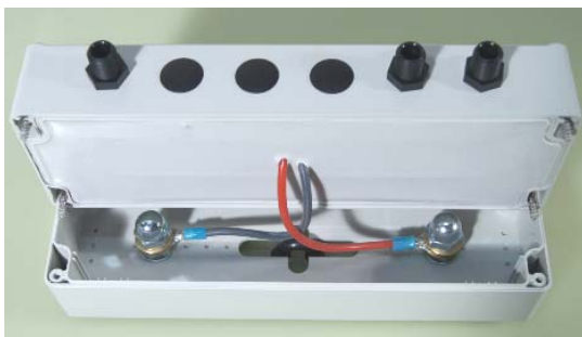
High Voltage terminals
