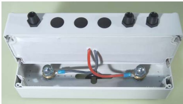
High Voltage terminals
